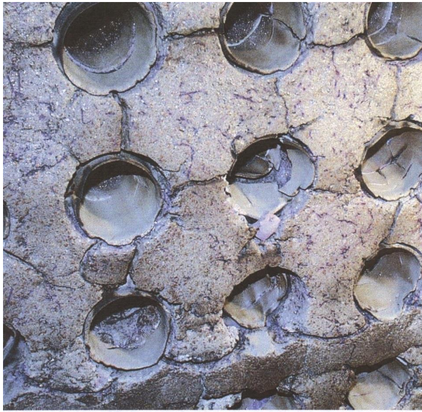
Figure B - Example of Ferrule Damage Due to Excessive Operating Temperature
