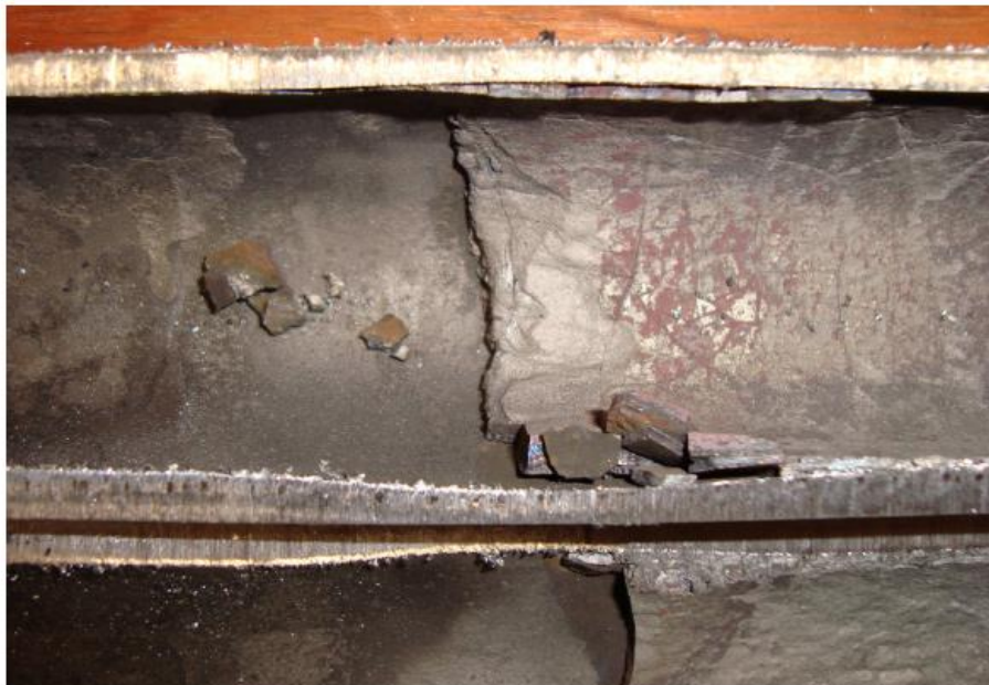
Figure H - Corrosion at end of ferrule due to water side fouling
