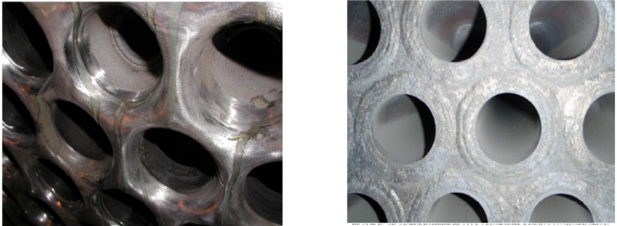
Figure D – Severly Corroded Original and Non-Corroded Replacement WHB Tube Sheets
