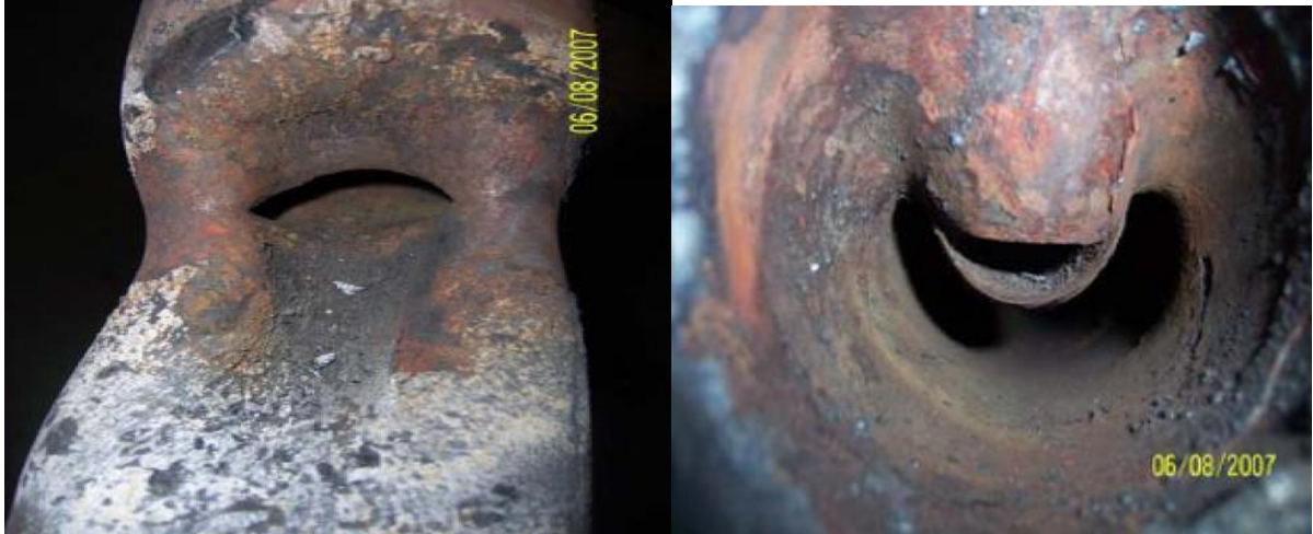
Figure G - Tube Collapse at End of Ferrule Due to Steam Blanketing Condition OD View on Left and ID View on Right
