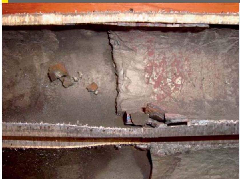
Fig 4: Corrosion at end of ferrule due to water side fouling
